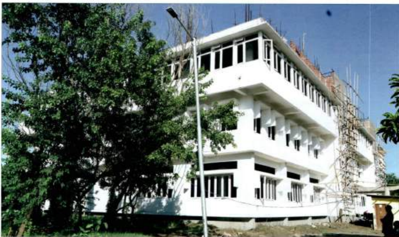
CIF and Drug Development centre Building at the final stage of completion.
