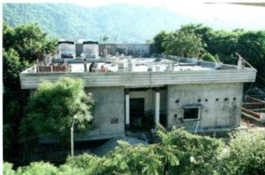
The sophisticated GLP compliant Animal House Facility (AHF) Building is nearing completion.
