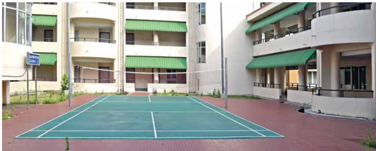
View of Students and Scientists' Home after Paving of Court Yard, Chajja projection and making badminton sports surface
