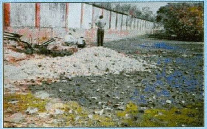
Contamination due to leakage and seepage of crude oil at Rudrasagar
