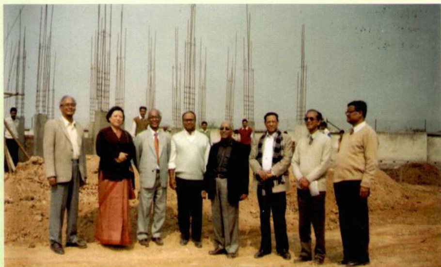
CONSTRUCTION SITE OF IASST at Boragaon in the year 2002 (Picture taken on 7-2-2002)
